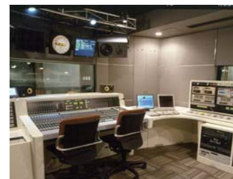
Television Broadcasting Studio Nittobo engages in the design and construction of acoustic studios.
